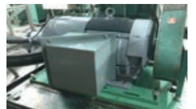
Installed take-up inverter motor
